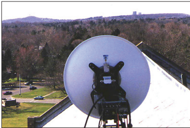
Figure 2.30 Microwave paths are often affected by trees and foliage that are either directly or even peripherally in the path. (Source: Tim Stoffel)
