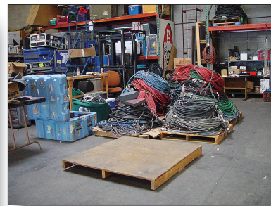
Figure 2.47 Various cable runs, mostly originating from the truck, must have lengths and amounts determined. If the truck being used doesn't have the necessary lengths, additional cable must be shipped to the site. Most large production trucks carry well over 100,000 feet of cable.
